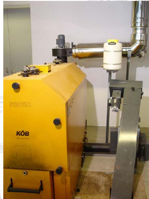
Thermal use of wood chips
