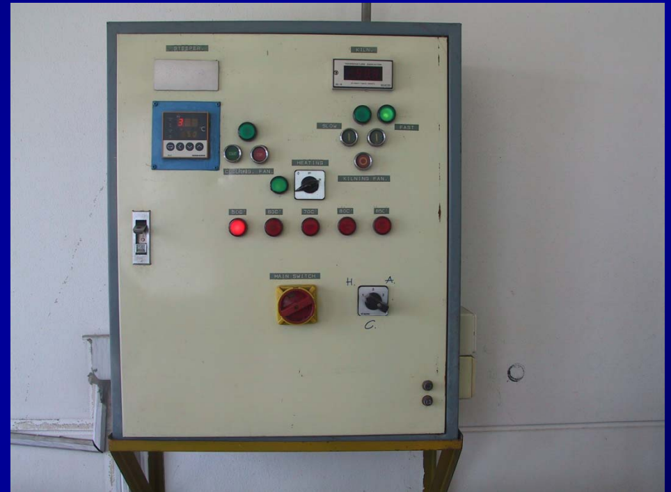
Temperature controlling panel
