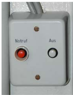
Emergency system in the institute
